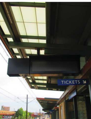
Variable Message Sign (VMS) (METRO Green Line shown)
